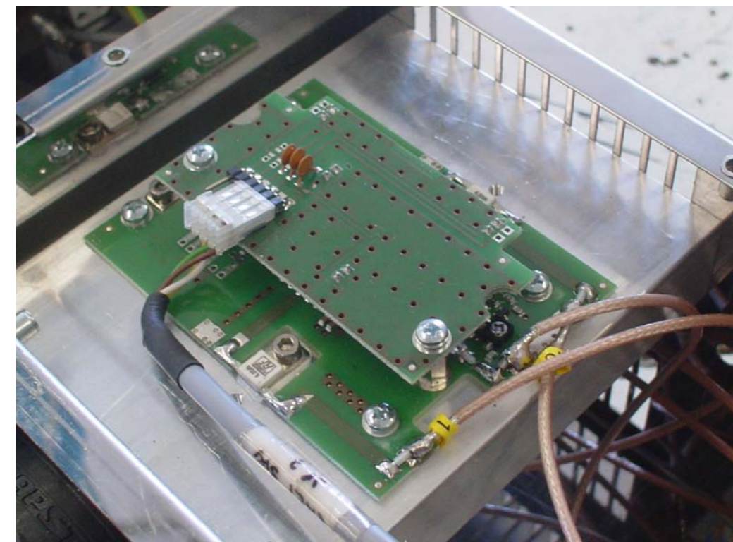
Exciter RF switch
